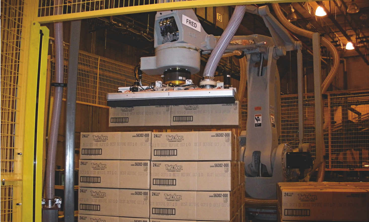
The robotic palletizing cells at Y&S pick cases from infeed conveyors fed by a main conveyor trunk line coming from the plant's packaging lines. Cases of the firm's candy products—Twizzlers, Nibs, etc.—range in size from 3.1x5.3x9.9 in. to 15.1x16.4x26.5 in. and weigh as much as 62.2 lb. Of the 149 active cases, 125 are column-stacked patterns and 24 have top layers rotated 180 deg to interlock the load.
